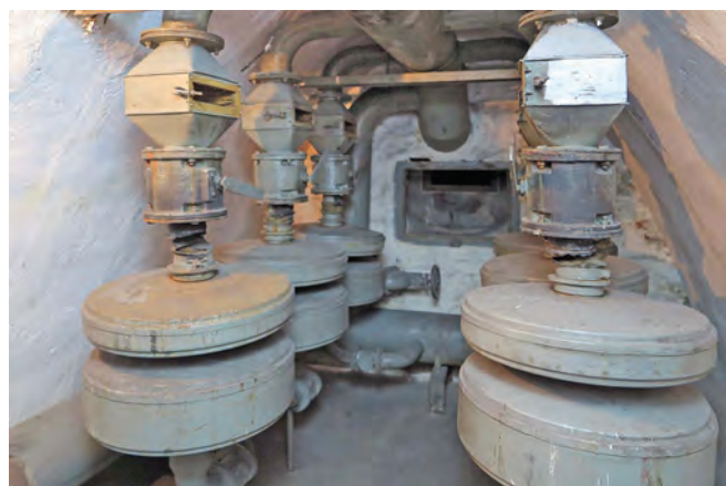
Filters within the Tamariska Shelter within the air-handling room
